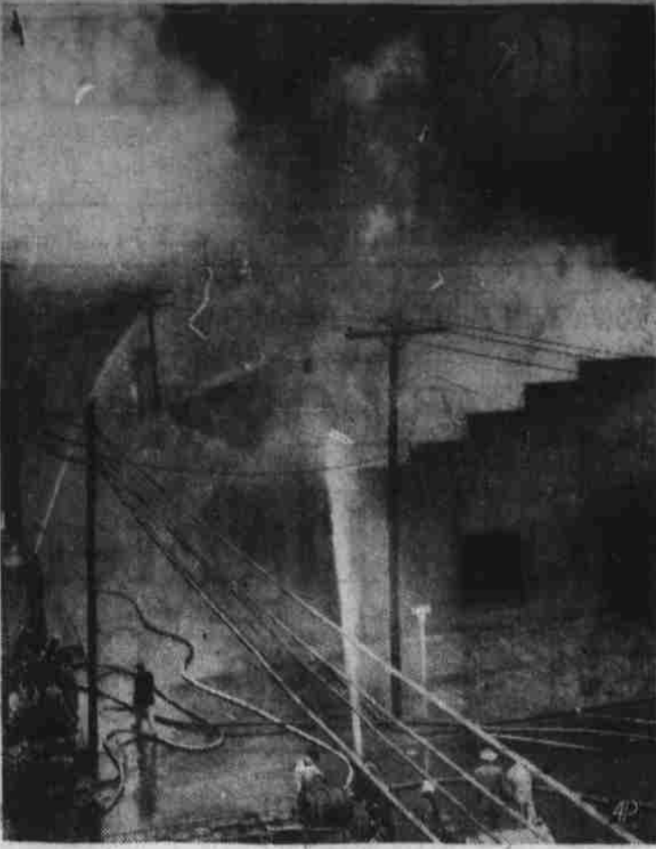
Firemen battle futilely against flames sweeping through the plant of the Kendall Medicine Company and an auto parts firm at Shelby. Damage was estimated at more than $350,000. Medical stocks destroyed included valuable packages of rare drugs. No one was injured. (AP Photo).
