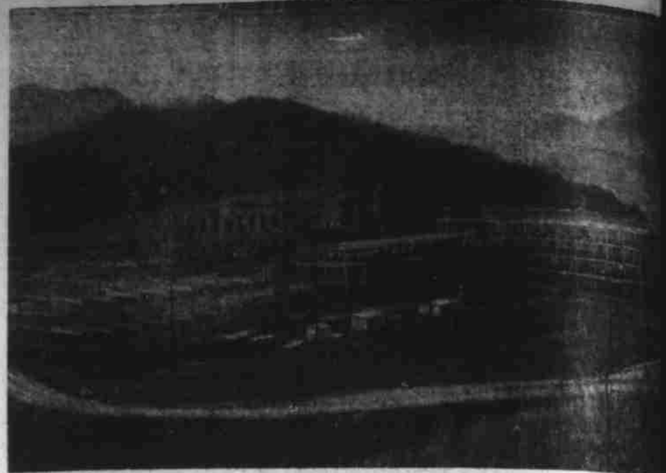
The new Library (left) at Western Carolina Teachers College is fast taking shape, while tons of steel framing being erected. On the right is the framework of the new science building.
