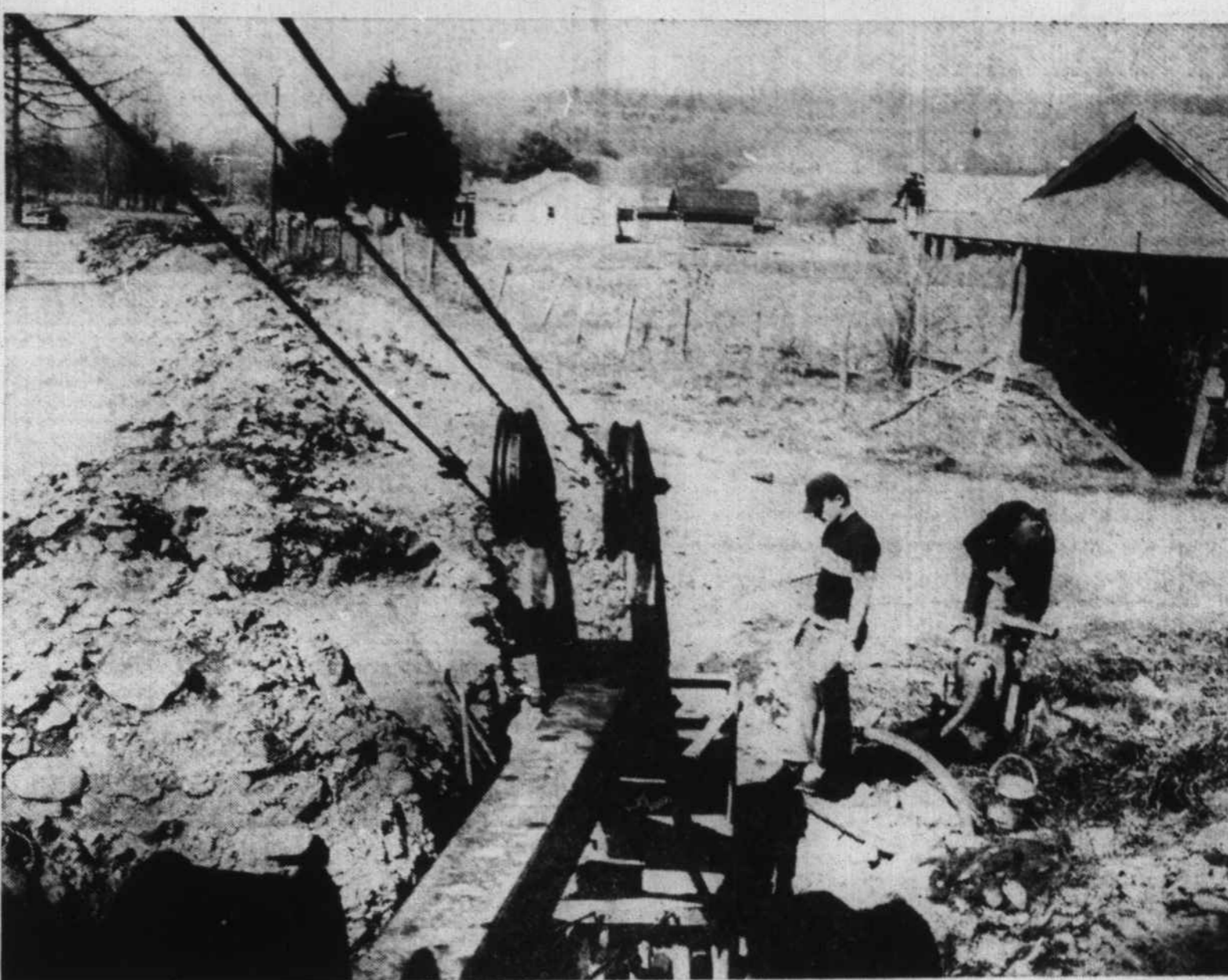
Workmen are pictured preparing to lay the new water line to service Waynesville's water needs. The line, which is a part of the $300,000 improvement in Waynesville's water service, will be 12 inches in diameter and will run 9500 feet. Another line, 10 inches in diameter, will run about 850 feet. Town officials are now awaiting complete plans and specifications for a modern filtering plant, being prepared by a firm of engineers. (Mountaineer Photo.)
