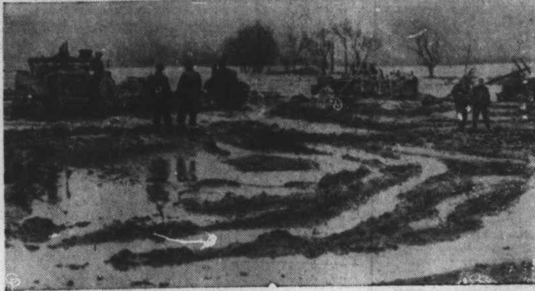
CIVIL DEFENSE WORKERS man tractors and bulldozers as every available piece of heavy equipment is put into use to strengthen the levee south of Yuba City, Calif., threatened by the Feather River Raging torrents are bearing down on the mud barriers that protect the city, which is still attempting to dry out from floods that swept the area in December, taking a toll of 33 lives. (International Soundphoto)
