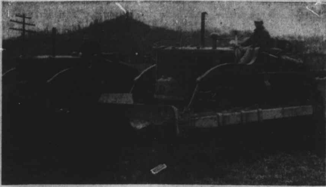
HUGE BULLDOZERS are shown here moving the first of 13,000 yards of dirt for the Unagusta plant. These machines started in a few minutes after the benediction of the formal ground-breaking ceremonies were completed. (Mountaineer Photo).
