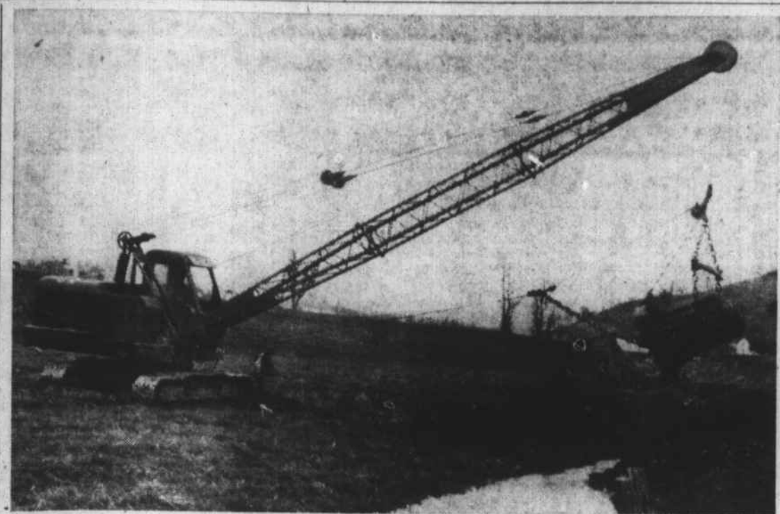
DREDGING OPERATIONS to widen, deepen, and straighten 3.775 feet of Raccoon Creek through the Mountain Experiment Station and the John Morrow farm in Ratcliffe Cove are scheduled to be completed this week by G. H. Bishop of Asheville, shown here operating his crane. The project was carried out to improve drainage on the test farm and the Morrow place.
