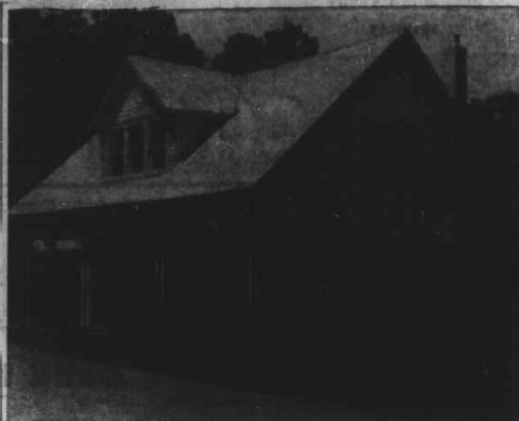
OWNERS OF THIS HOUSE on Daisy Ave.—Mr. and Mrs. William Lenoir—have been commended by the Waynesville cleanup campaign committee for their work on the dwelling after it was badly damaged by fire on April 5. Considerable painting and repairs have been done on the east side of the house, where the blaze broke out. (Mountaineer Photo).
