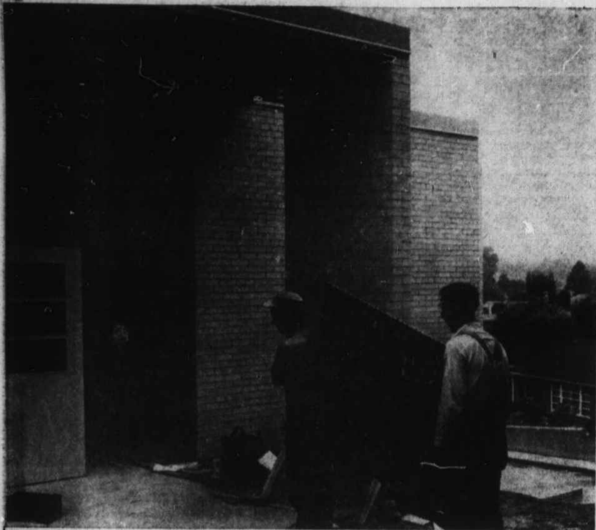
GO THE SLATE blackboards in the new $145,000 St. John's School, which is nearing completion here. The workmen are entering the Church Street door of the building, which will serve the elementary grades of the school. (Mountaineer Photo).
