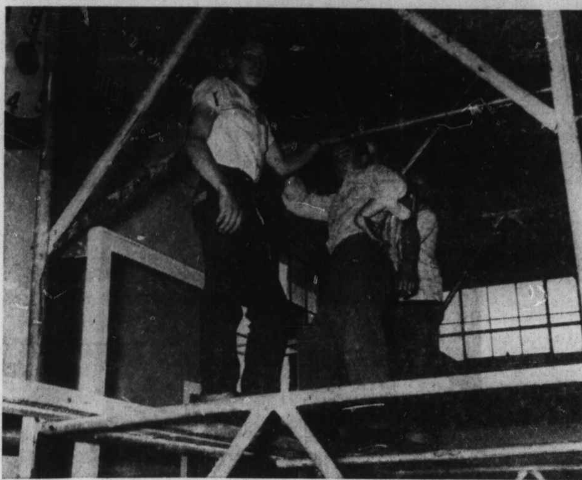
NEW GLASS BACKBOARDS were installed in the Fines Creek High School gymnasium this week by this group of students and several adult workmen. Other work being done at the school includes the installation of a new boiler and laying of additional concrete walks on the school grounds. (Mountaineer Photo).
