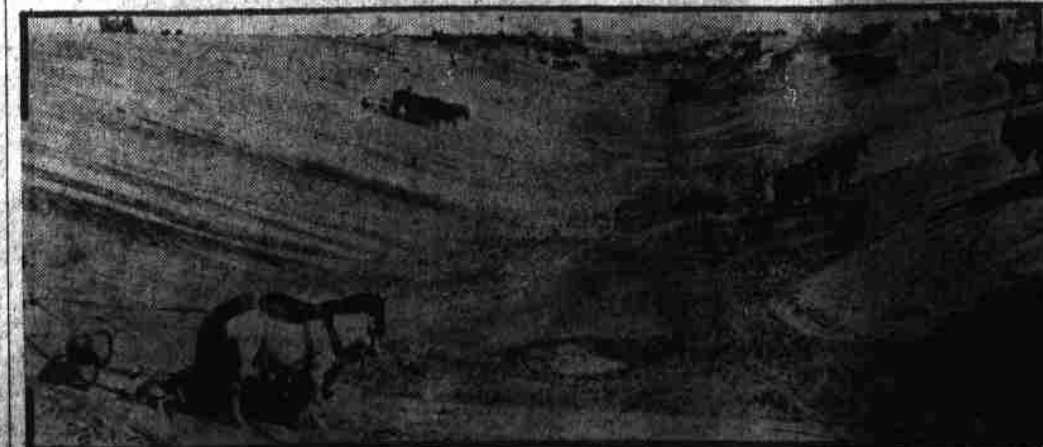
One hundred four-horse teams are here busy on one section of the All-American canal which will replace the main now serving California's Imperial valley.
