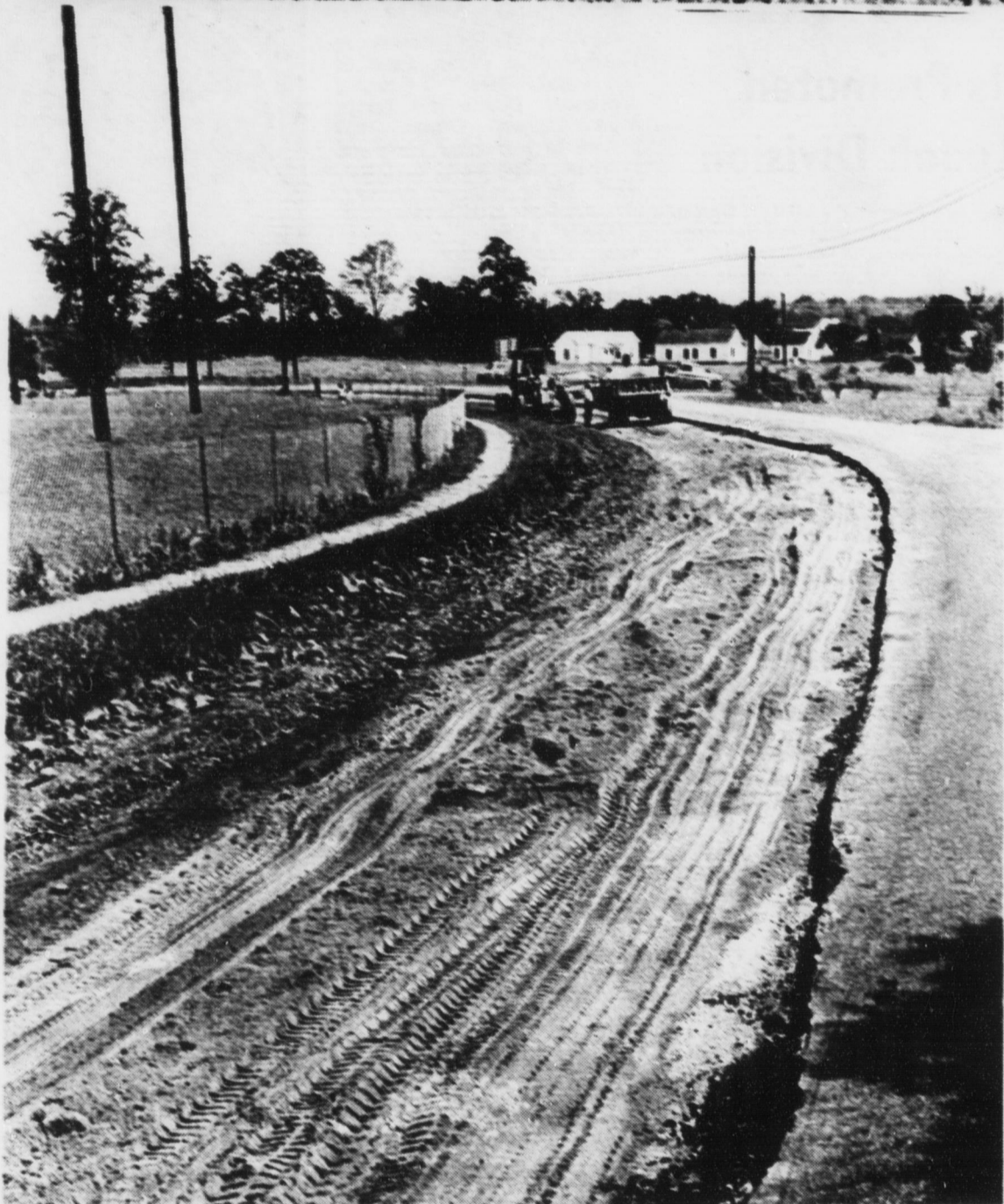
Work began this week on the ball park curve. Upon completion, the inside of the curve will be raised 18 inches in hopes of preventing hazardous driving this winter. In winters past, we have printed pictures showing cars in the ditch all around this famous curve. In just a few more months we'll know whether or not this was an improvement.
