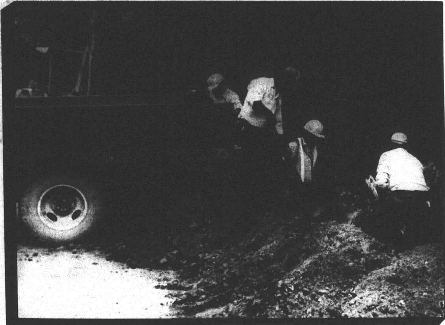
Helping city SYEF employee Orlando Tillman lends a hand as Raeford City workers lay pipe.
