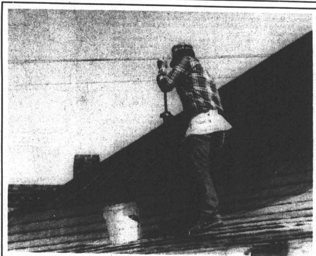
Up on the roof Local roofing contractor Richard Odom expertly covers a portion of the old Aberdeen-Rockfish Depot roof with dark green paint. Odom repaired and painted half the roof before running out of
