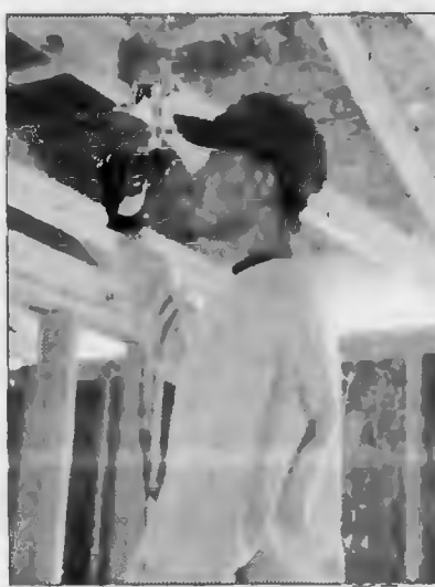
Pinehurst firefighter Cy Kirk installs a sprinkler in the Habitat House here.
