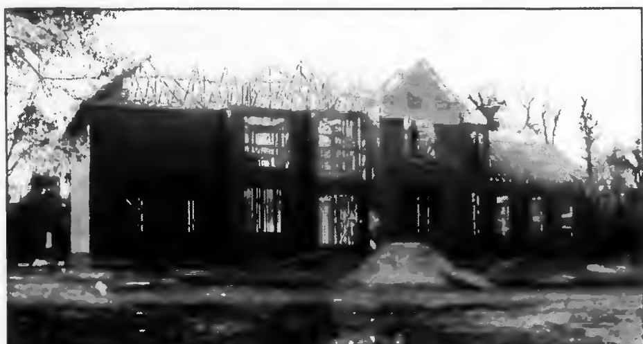
A 3,500 square foot house, which will be surrounded by a brick wall, is being built on North Main Street by pop star Michael Jackson.
