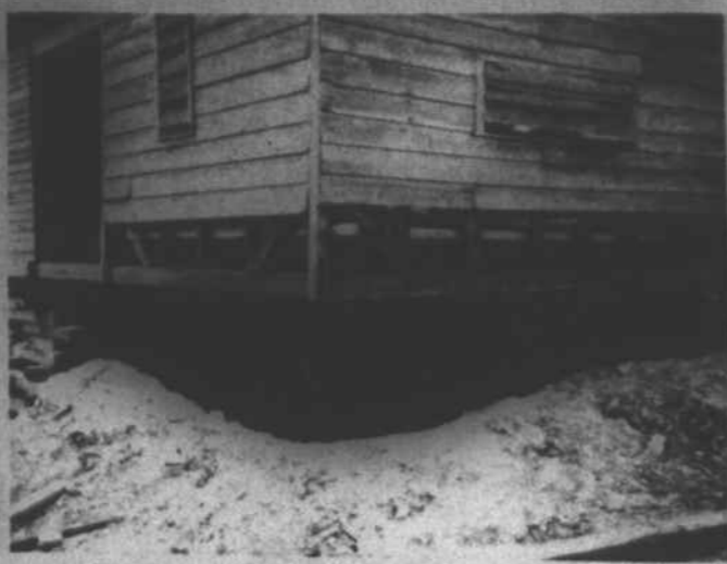
Under the kitchen and pantry, the wine cellar, with 12 inch brick walls, will be restored, and the original brick will be used. It is interesting to note that only a very few of the joists under the house were in bad condition. One of them was under the kitchen. The house is now supported by steel beams, waiting to be replaced on the brick pillars which are being repaired and restored.
