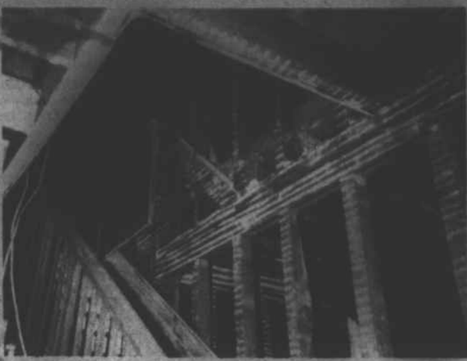
Inside views of Liberty Hall. The above picture shows where all plaster and lathes have been removed and the woodwork around the windows and door facings have been sanded. This is a scene on the second floor. In the picture below are the stair steps going to the second floor. Note in the center of the picture where the corner is braced. The corner brace is mortised and pegged into the long timber which goes all the way from the bottom of the house to the top, approximately twenty-two feet long.
