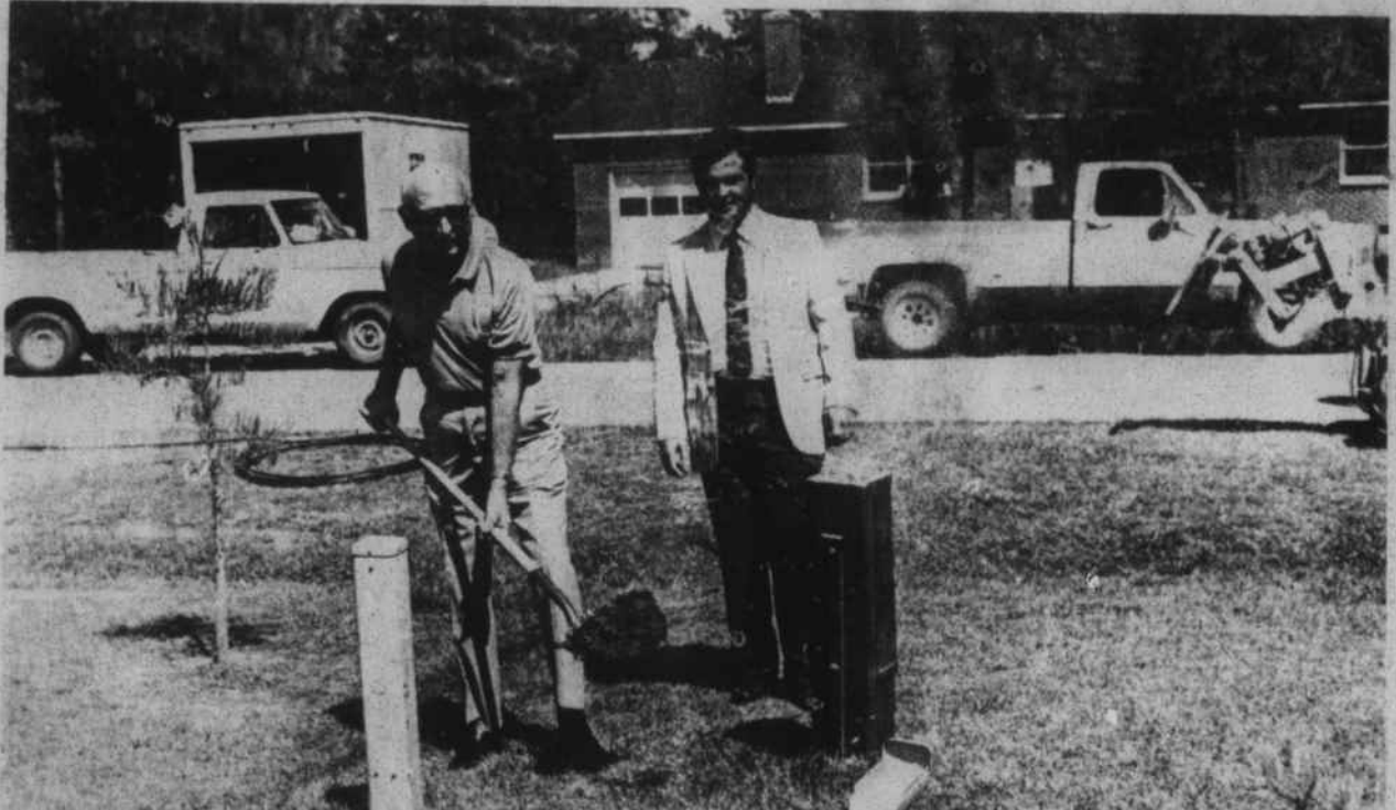
TV CABLE GROUDBREAKING - Warsaw Mayor Sam Godwin and Clear-Tel Cable TV President Michael Hanno turn the turf as Warsaw's TV cable system begins its underground journey to Warsaw homes.
