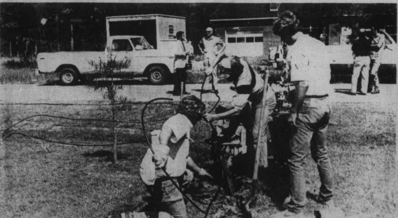
CABLE TV WORKMEN begin plowing in the TV cable on Dogwood Drive in Warsaw. Home installations are expected to begin in December.
