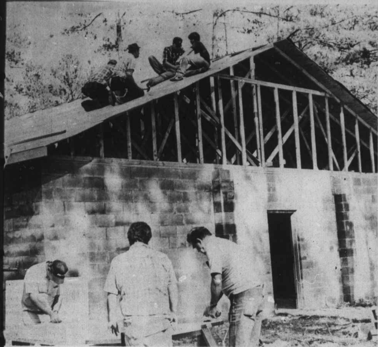
DUPLIN LAW ENFORCEMENT BUILDING TAKING SHAPE - Duplin law enforcement officers are putting on the roof of their new building located north of Kenansville. Most of the work has been done by officers off duty or paid
