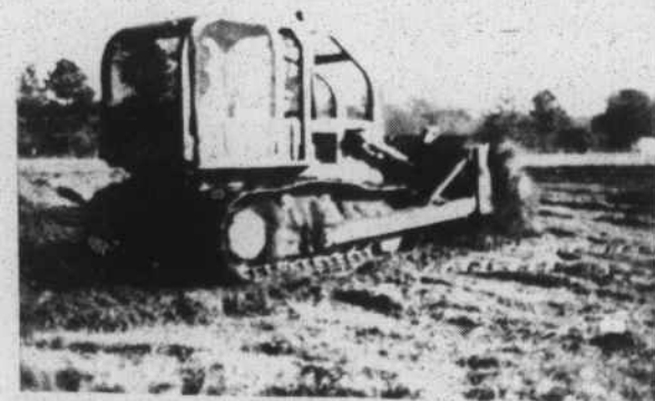
BULDOZER WORK BEGINS - Bulldozer work began on Friday to level a lot so construction can begin on the new First Baptist Church in Pink Hill. The 2,880-square foot structure is scheduled to be completed by late April. The location of the new building is on the corner of Stroud Road and Potter's Hill Road. The Rev. Tommy Tripp is the pastor. Pink Hill First Baptist Church was organized almost a year ago. The congregation is very appreciative of the use of the Pink Hill Veterans of Foreign Wars Hut for worship services since that time.
