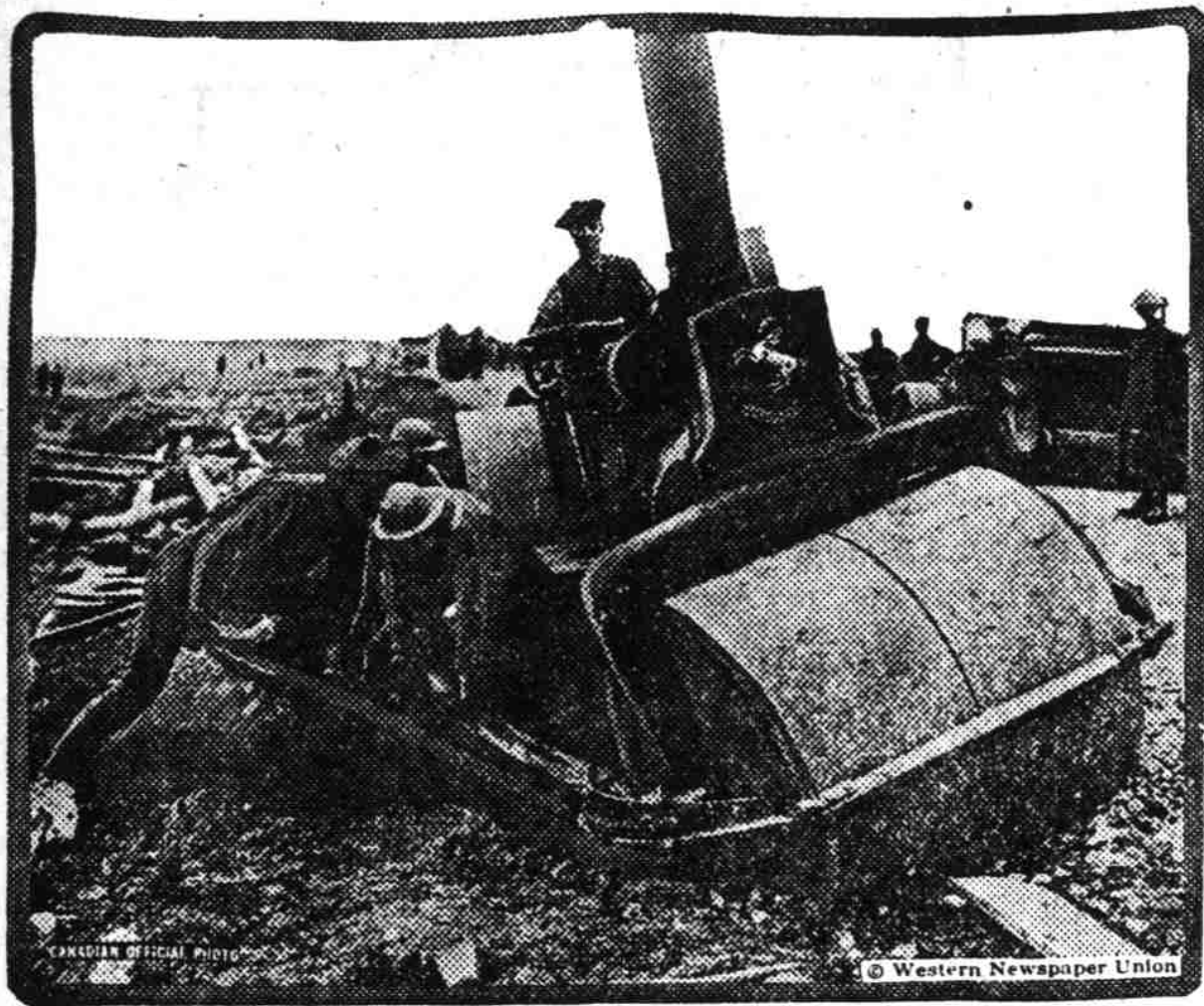
The engineers across the water are constantly busy making roads and reconstructing those that have been torn up by shells. Here is a roller that has got stuck in a ditch, and it takes husky Canadians like those you see to pry it back into place.
