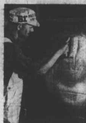
Circular scrub brushing spreads cement-water paint over wall dampened by a fine fog spray.
