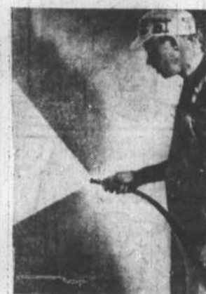
Each coat is cured by keeping wall damp with fog spray for 24 to 48 hours to prevent hair cracks.
