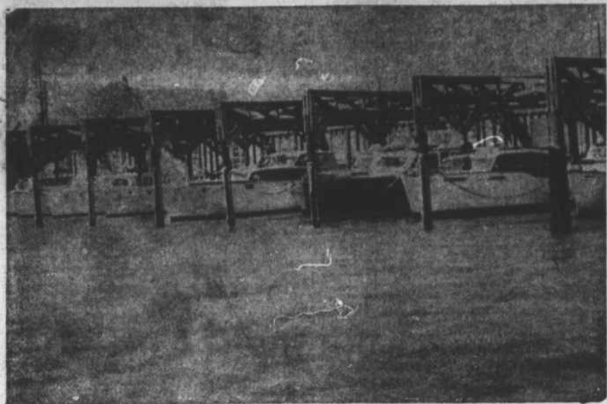
The boat shed at the Morehead City Yacht Basin lost its roof Saturday night. None of the boats pictured here was damaged.
