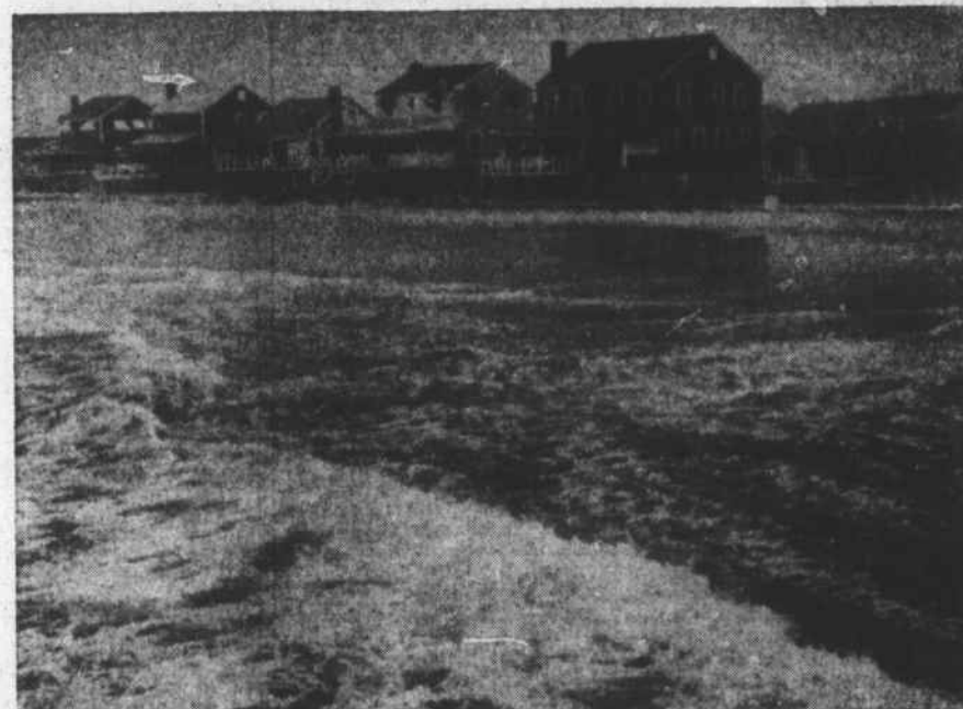
The creosoted wood piling seawall constructed in front of these cottages at Money Island proved its worth during Helene. At no time during the storm did breakers go over the wall.
