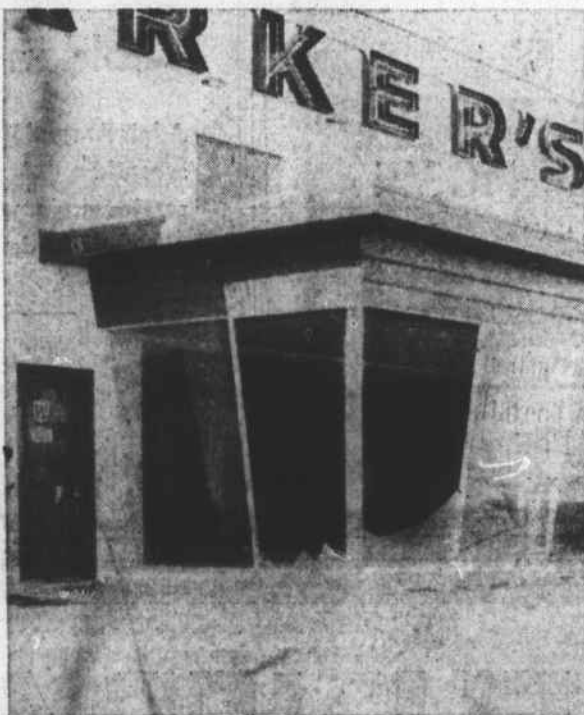
Parker Motors, along with several other Morehead City businesses, lost considerable amounts of plate glass. This picture shows the east side of the building.
