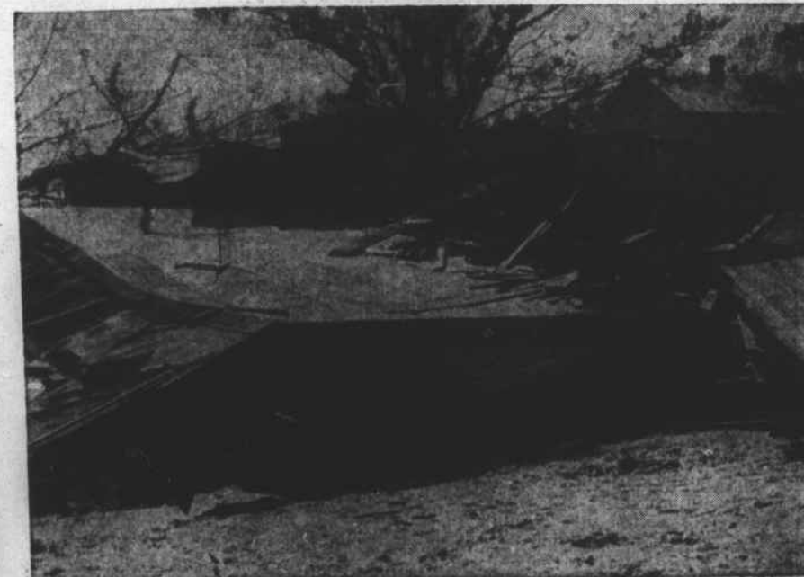
Helene lowered the boom on this house on Cedar Street, Beaufort. The walls collapsed and the roof settled directly on the foundation.
