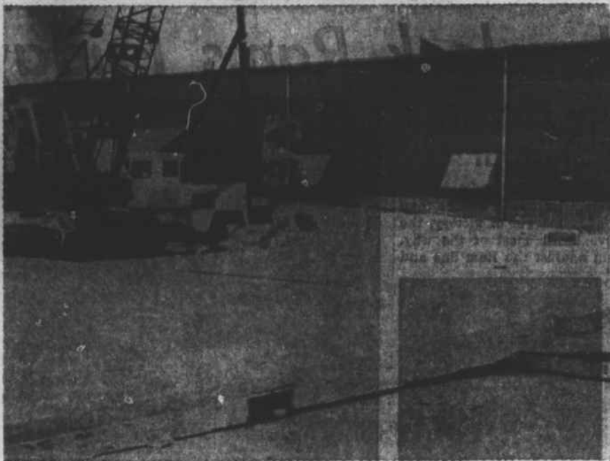
These masonry wall panels in the warehouse under construction at state port were flattened during hurricane Helene. The crane in the background is clearing away the rubble.
