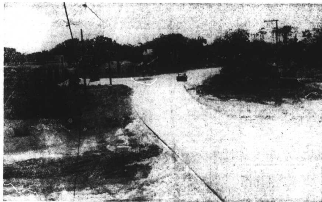
Bulldozers this week have been clearing the way for the new dual lane highway into Morehead City. This shows the highway just west of the Blue Ribbon restaurant, facing west. Felled trees are piled at either side of the present highway.
