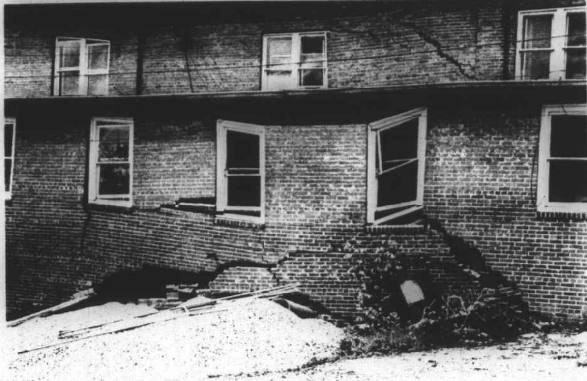
Rear Wall Of Murphy Carnegie Library Collapses
