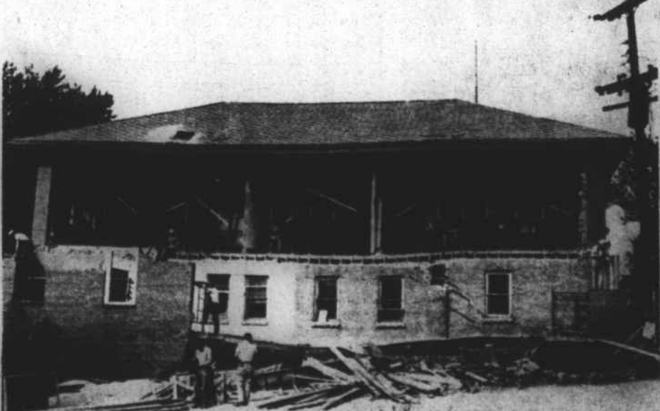
DAMAGED WALL of the Murphy Carnegie Library was being reconstructed this week. This work began the day following the collapse of the rear wall of the building. The wall collapsed has been blamed on heavy rains which followed extensive excavations in the basement of the building for a fire station to house Murphy's new fire truck. The rear wall will be replaced. A new fire station at the rear of the library is contemplated. This project has not been approved however by the Murphy town board, C. E. Johnson, town clerk, said. Smith and Jones Construction Co. have been employed by the town on an emergency forced account agreement. The extreme necessity of starting repair work immediately was brought about due to the hazards of the building collapsing further. (Scout Photo)
