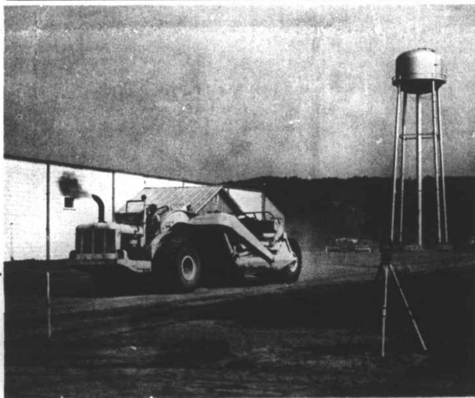
EARTH MOVERS BEGAN WORK Tuesday, June 23, at the Textured Yarn Plant at Peachtree on their thirty-two thousand square foot addition. This addition doubles the size of the original plant.
