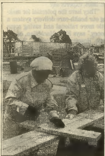
With the help of Kaboom, volunteers construct a playground in a low-income community in Washington.
