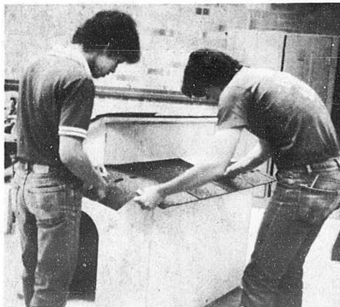
KERMIT BROGAN and RANDY WARD place the roof shingles to the shallow side of the salt box roof.
