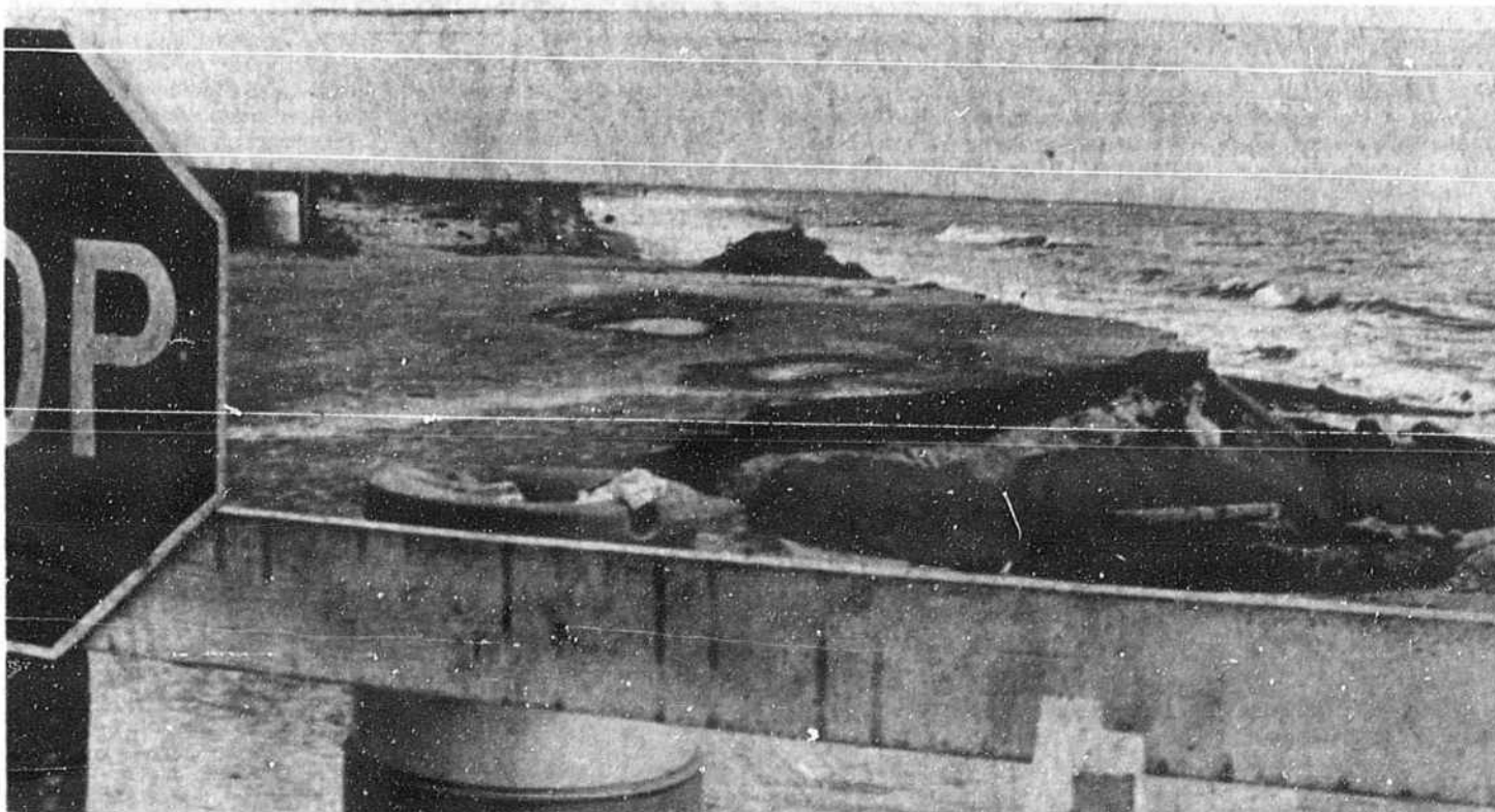
A PEEK THROUGH THE BARRICADE at the east end of Holden Beach reveals the cul-de-sac collapsed by high tides and rough seas recently. The east end of Ocean Boulevard may be the next thing to go, Mayor Kenner
