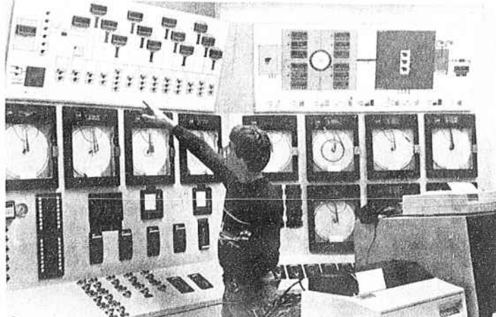
WATER PLANT TECHNICIAN David Rourke, of Stallotte, points to display panels in the main control
