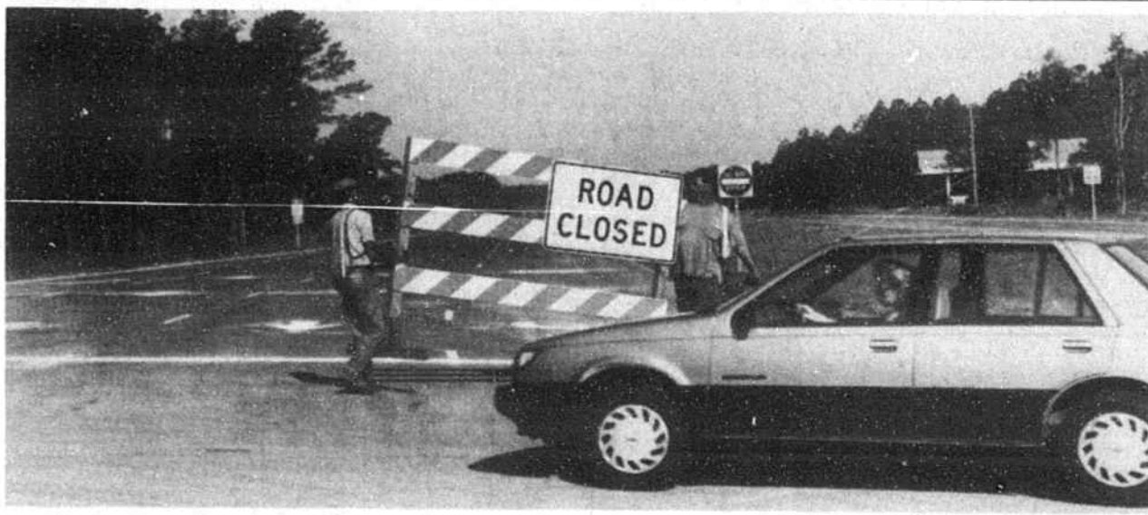
A ROAD CREW removes a barricade at the north end of the bypass last Wednesday, clearing the way for the first wave of traffic on the five-mile stretch.
