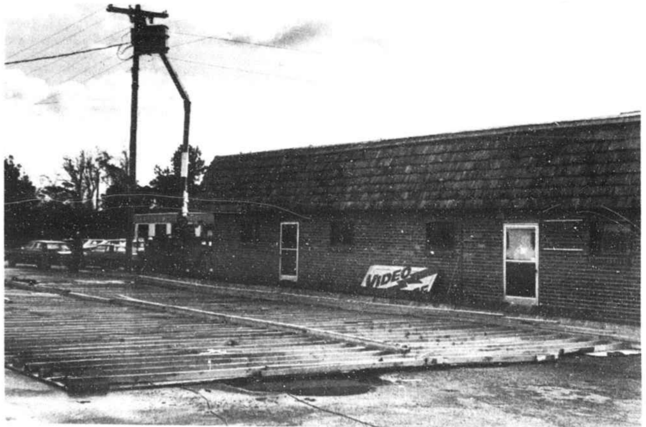
VIDEO VOLTAGE lost its roof in last Thursday's storm. Officials believe a downburst of wind lifted the roof off the building and left it upside down in the front parking lot. STAFF PHOTO BY DOUG RUTTER
