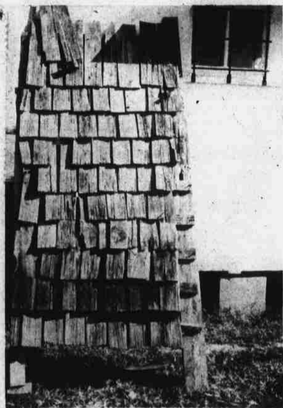
OLD SHINGLES — This section of shingles is over 100 years old. It was used on the Newbold-White House to replace the original ones which had probably begun to leak. The section is being used as a guideline for the shingles currently being made.
