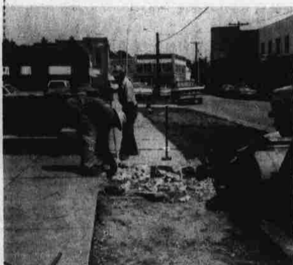
SIDEWALK REPAIR — These Town of Hertford employes work on replacing sidewalk section along Market Street in front of the Hertford Baptist Church. Sidewalk repair work has also been done on the sections in front of the stores on that street. (Newbern photo)
