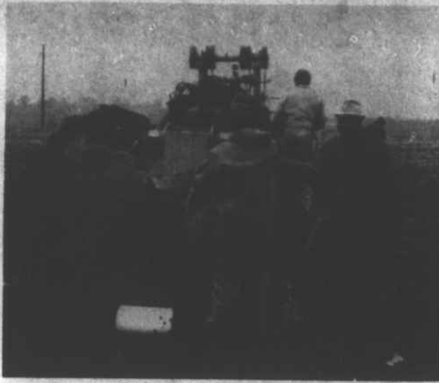
TILE SYSTEM BEING USED — J.B. Rountree's crew is shown installing tile on the William Charlie Roberts farm. Over 15,000 feet of tile will be installed in Perquimans County this spring. (SCS Photo)
