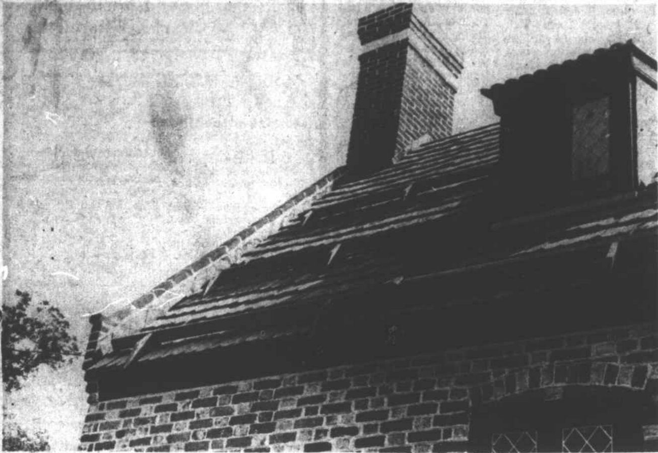
CLOSE-UP OF COMPLETED SECTION — This picture of the completed roof section on the Newbold-White House shows the shingle detail
