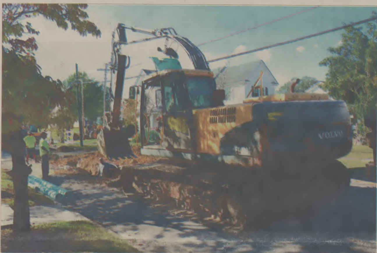
Heavy equipment excavates a hole in Market Street Monday as part of a project to replace aging sewer lines. The construction has forced the closure of some roads.
