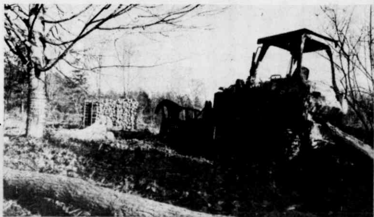
Heavy equipment, cut logs and cleared land where in December we had the Groundbreaking Ceremony.
