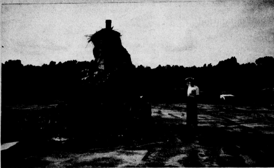
When we began, the pipe at the top of this mound was 2 feet BELOW GROUND LEVEL on the crest of a hill! Now, the mound stands above the flat site of the future athletic field as a dramatic indicator of how the site has been reshaped.
