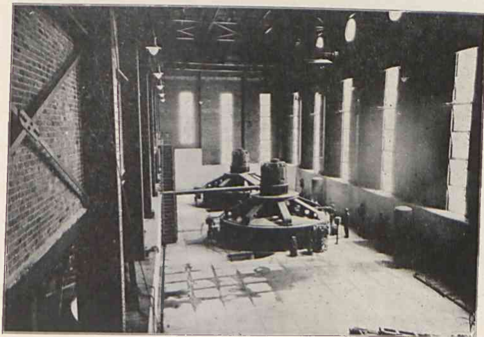
INTERIOR VIEW—YADKIN FALLS POWER-HOUSE
