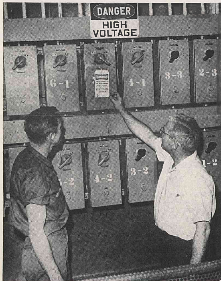
RED TAG FOR SAFETY —Ed Taylor, maintenance foreman, right, explains to Roy Chastain, Shop, importance of an attached red tag to an electrical switch in the "off" position. This is a standard safety measure practiced while work is being done on electrical circuits, machinery and other equipment where there is danger of accidental or careless starting of the machinery. When deemed advisable the switch lever may be padlocked as an extra precaution.
