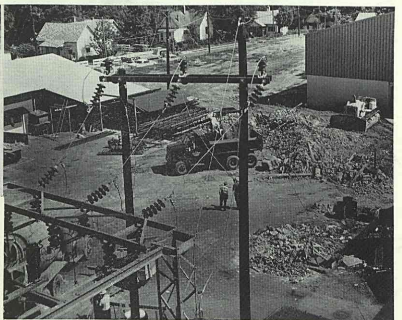
Right: Workmen cleared brick and rubble, while others were busy at constructing new outdoor electric station (portion at left in picture). This one, at site of old welding shop, will have greater capacity than its predecessor. New installation will be teamed with existing station off Vance Street.
