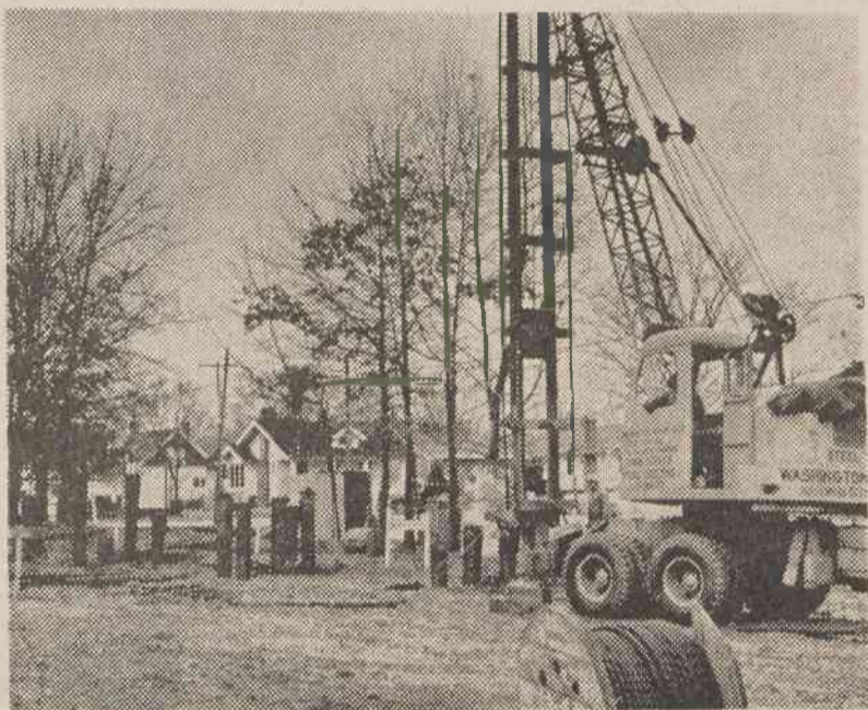
DORM WORK BEGINS —The large pile driver shown above was busy this week on the site of Atlantic Christian's new men's dormitory. Piles are being driven into the ground on the site to provide a foundation for the structure. (Collegiate Photo by Claude Anthony)
