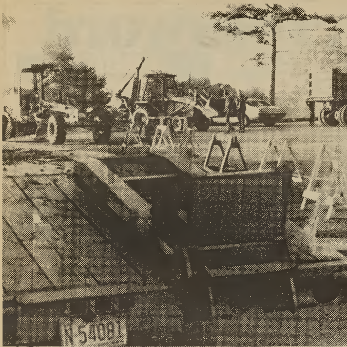
Dozing Dozers: Heavy equipment occupies part of the Carmichael Building parking lot as the first day of construction on the new lower lot ends.
