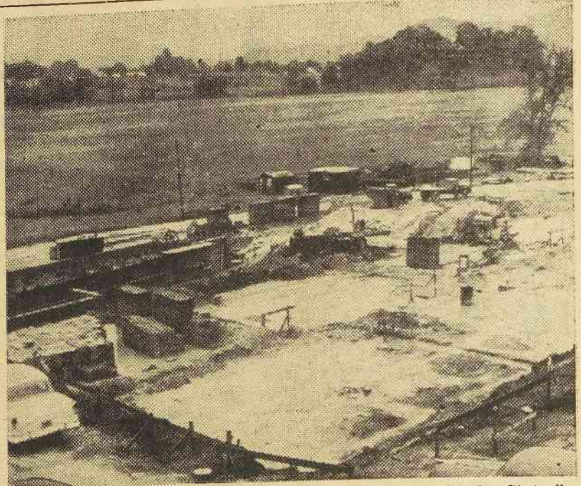
"TO BUILD THE FINEST structure of its type in the States", is the ambition of Mr. J. D. Jamerson, superintendent for the J. A. Jones Construction Co., as he labors to complete the new Campus Center building by early 1957. The photographer is standing near the northwest corner of the foundation looking in a southeasterly direction.
