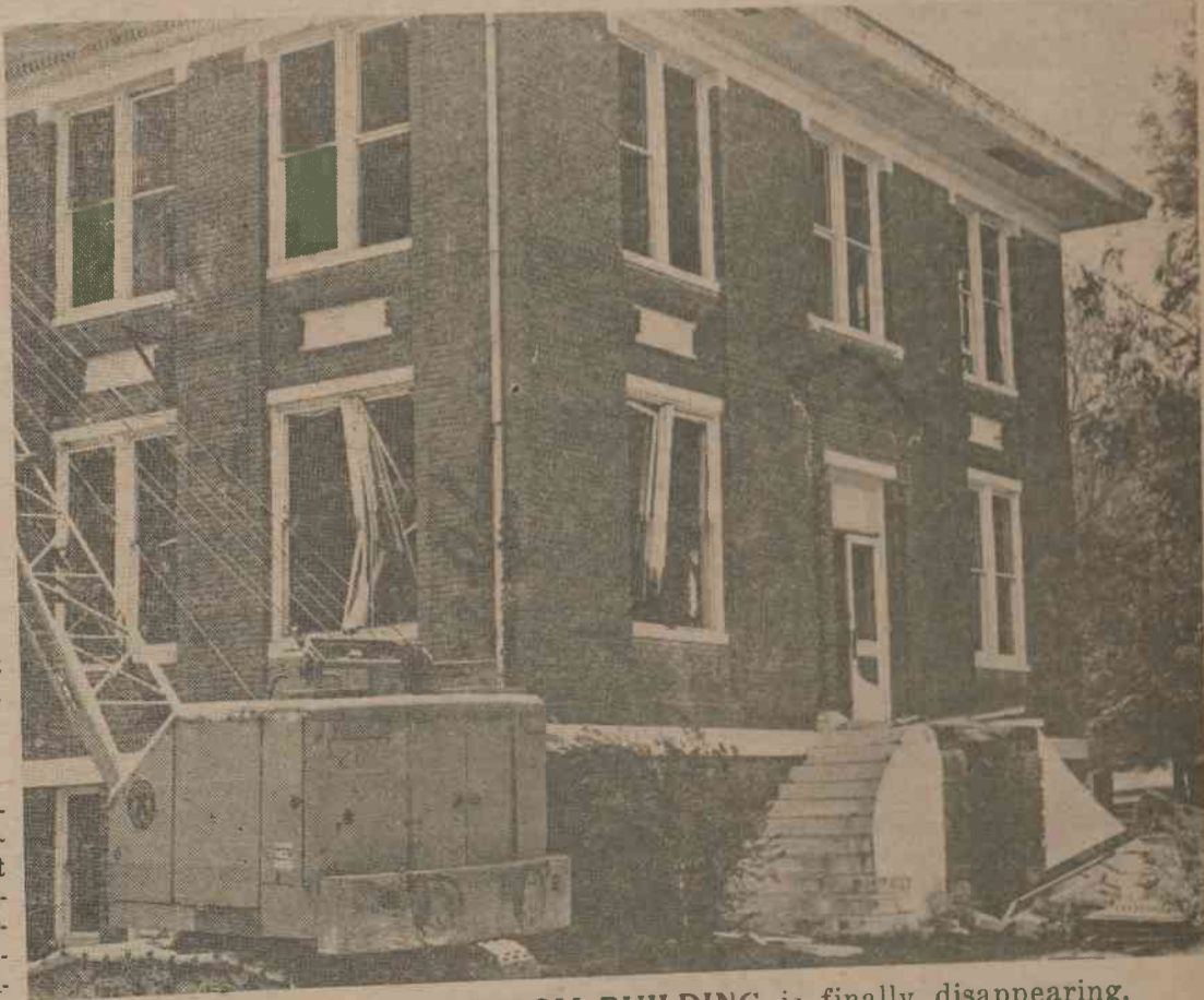
THE OLD CLASSROOM BUILDING is finally disappearing, brick by brick, from the College Campus, as demolition work has begun.
