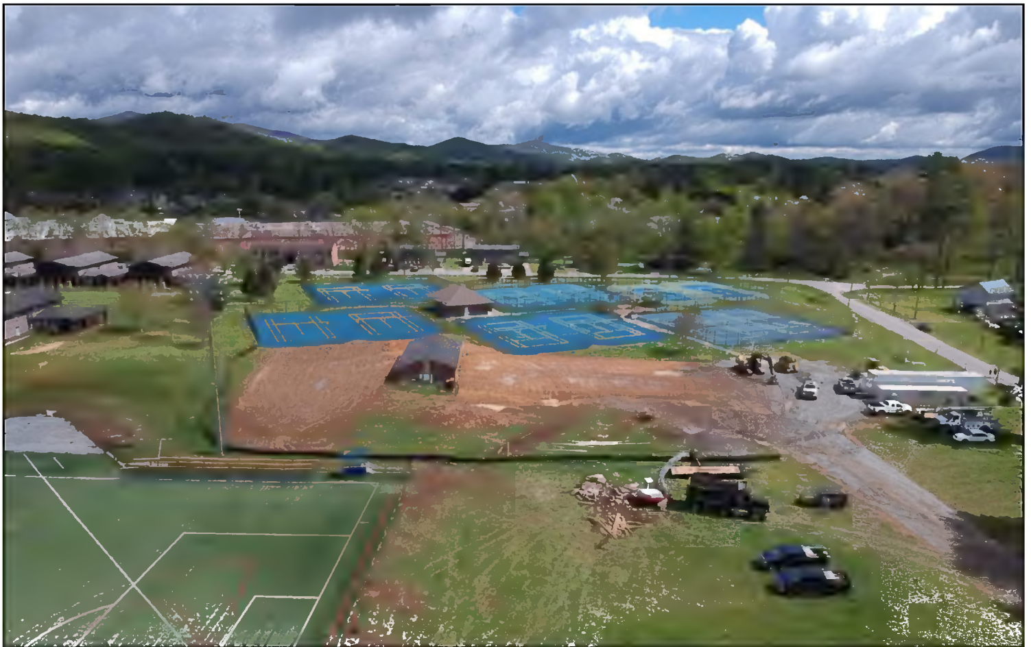
An aerial view of construction on the new BC athletics field house on the Brevard College campus. The new field house will include offices, classroom and meeting space, and locker room facilities for student-athletes in five team sports. It is scheduled to be completed in time for the fall 2020 semester. For a short video showing the construction of the facility, visit www.youtube.com/watch?v=gMxBbOxtkHw .
