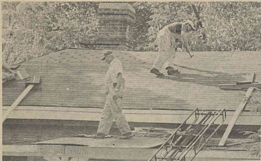
Carpenters work on McFarland House. Renovation of the interior will begin soon.
