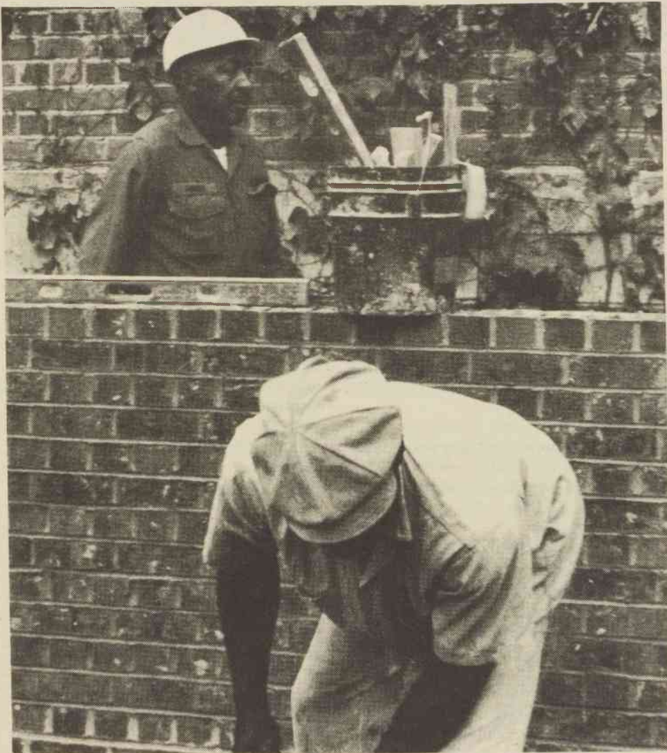
Although these two men are constructing a ramp on the side of Murphy Hall, on campus, for the handicapped, they differ greatly in age and years of experience. Larry Everette, 23, from Burlington, (bending down) has been working with his bricklaying company for five months. But Thomas Purefoy, 54, (behind the wall) from Carrboro, has been in the bricklaying profession for 25 years.
